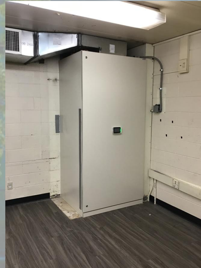
New Vertical Unit Ventilator in room 106
